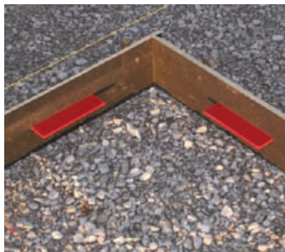
Figure 6-20. Unlike round dowel bars, plate dowels can be positioned near slab panel corners at construction joint intersections to provide load transfer at corners. Dowels have either a 45 degree taper (above, from ACI 302.1R) or cushioned sides (right) to allow unrestrained movement. (Photo courtesy of McTech Group, Inc.)
