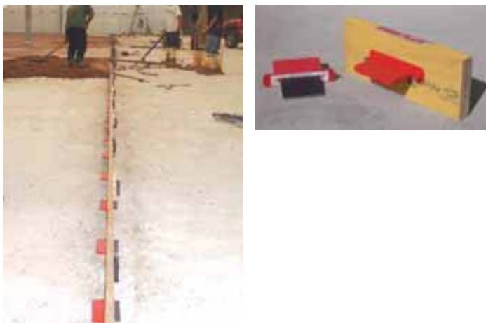
Figure 6-19. Plate dowels can be properly positioned in construction joints using either slotted forms or pocket-forming inserts. (Photos courtesy of McTech Group, Inc., and Greenstreak Group, Inc., and PNA Construction Technologies.)
