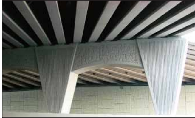
Photo Courtesy of Gresham, Smith and Partners
