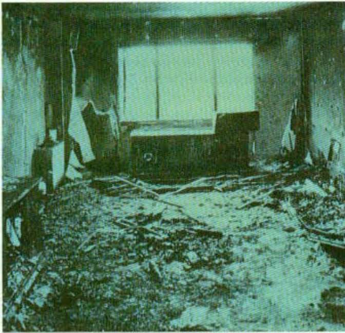
Although the contents of this dwelling unit were destroyed by fire, the concrete walls and ceiling prevented the fire from spreading beyond the unit of origin.
