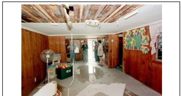
Source: Federal Emergency Management Agency, photograph taken by Dave Gatley of FEMA.
