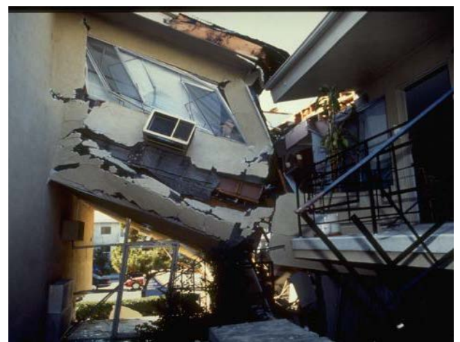
Source: Federal Emergency Management Agency Earthquake damage to personal property.
