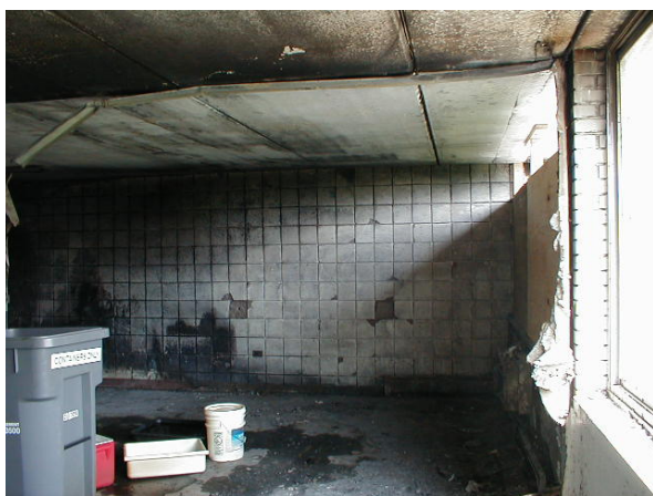
Source: Northeast Fire Safety Construction Advisory Council Fire resistant non-combustible materials contain fires, minimizing fire and smoke damage. This damage resistance allows portions of the buildings to simply be cleaned, painted, and reoccupied rather than completely re-constructed.
