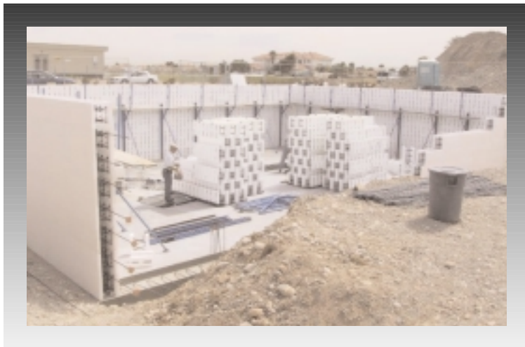
Ease of construction means ICF walls go up quickly. Merlin Contracting was so impressed, they recently became an Arxx dealer.
