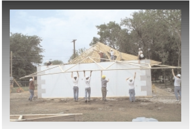
Trusses are being set on the 1,260-square-foot home being constructed by Oklahoma's largest contractor, Manhattan Construction, with the support of the City of Tulsa, American Lung Association of Oklahoma, American Institute of Architects, and Tulsa Project Impact.
