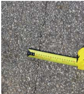
Fig.1. Narrow reflection crack
