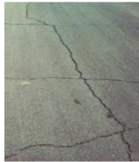
Fig. 2. Wide reflection cracks
