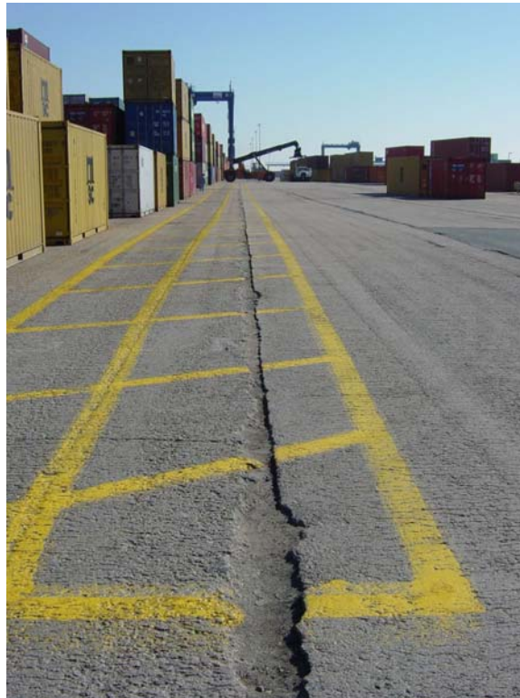
Fig 3. Longitudinal joint spalling at Conley Terminal (RCC is 17 years old).
