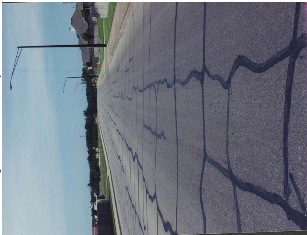
b) Soil-Cement Section (Excessive shrinkage of the stabilized base results in block cracking. This is initially cosmetic but can lead to secondary structural problems and loss of riding quality)
