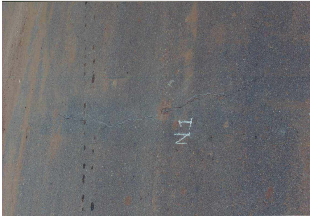
(b) Neuburg (only crack in section)
