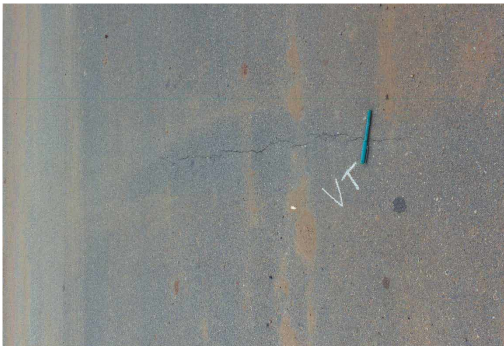
a) Von Trapp (Two cracks in 455-ft section)
