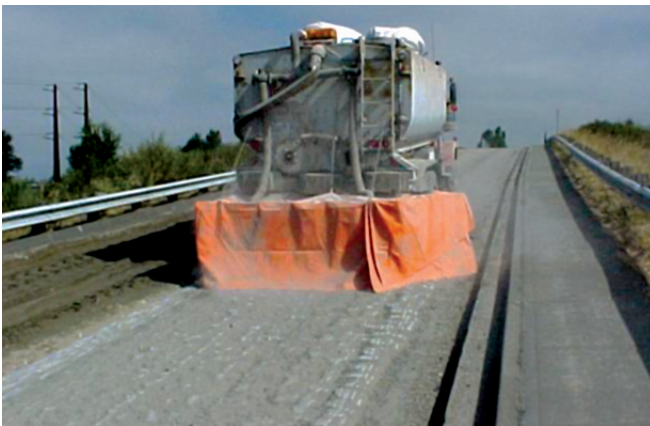
Figure 3.2. In mixed-in-place construction, cement is uniformly distributed over the area to be processed.
