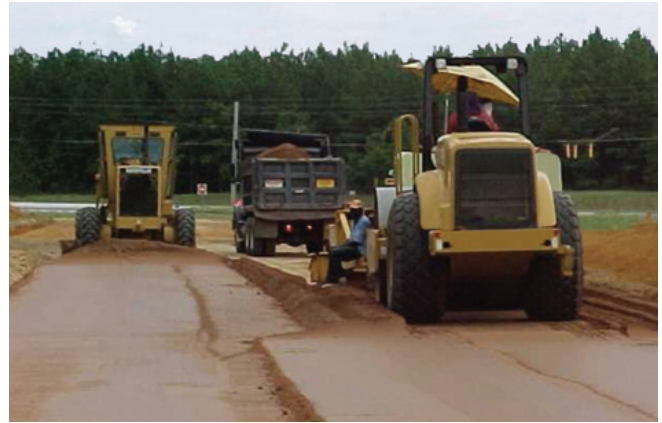
Figure 3.5. Soil/aggregate spreading operation working in staggered position across roadway to minimize longitudinal cold joints.
