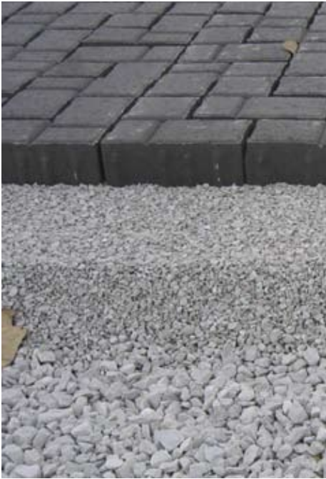
Figure 1. The permeable pavers, bedding and base are shown here. Not shown is the subbase or the permeable stone material that fills the joints.
