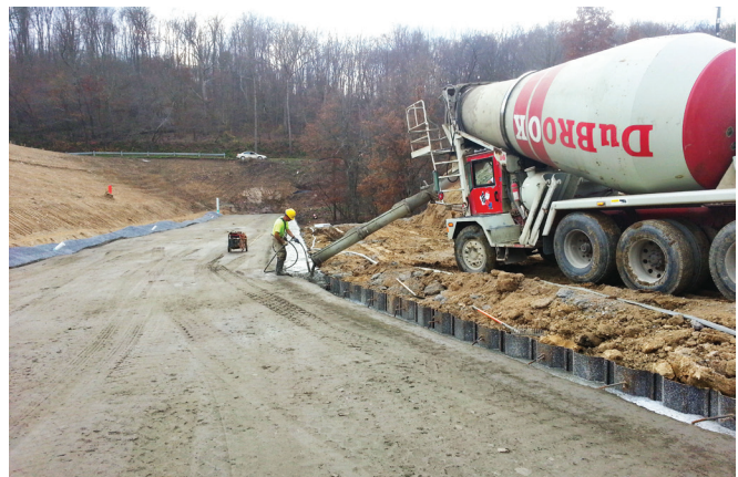
FIGURE 6-32. Backfilling steel sheet pile cutoff with conventional concrete (Lake Oneida Dam, PA).
