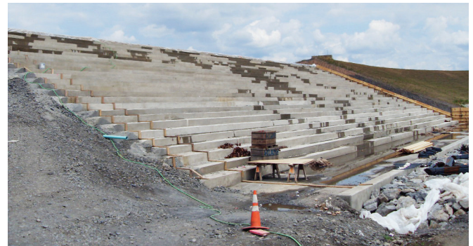
FIGURE 6-12. Formed RCC chute (Toby Creek Impounding Basin, PA), courtesy of KC Construction.
