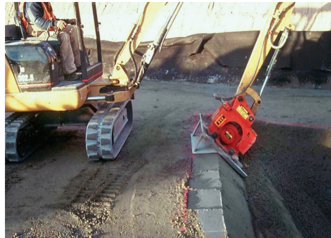
FIGURE 9-17. Vibratory plate compactor attachment on hydraulic excavator used to compact exposed RCC face.
