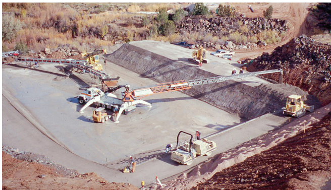
FIGURE 6-25. RCC spillway prior to installation of fuse gates shown in Figure 6-24 (Black Rock Dam, NM).
