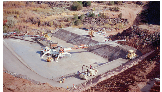
FIGURE 9-9. “Super Swinger” conveyor delivery system.
