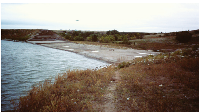
FIGURE 2-4. Downstream (top) and upstream (bottom) views of combined principal and auxiliary spillway (He Dog Dam, SD).
