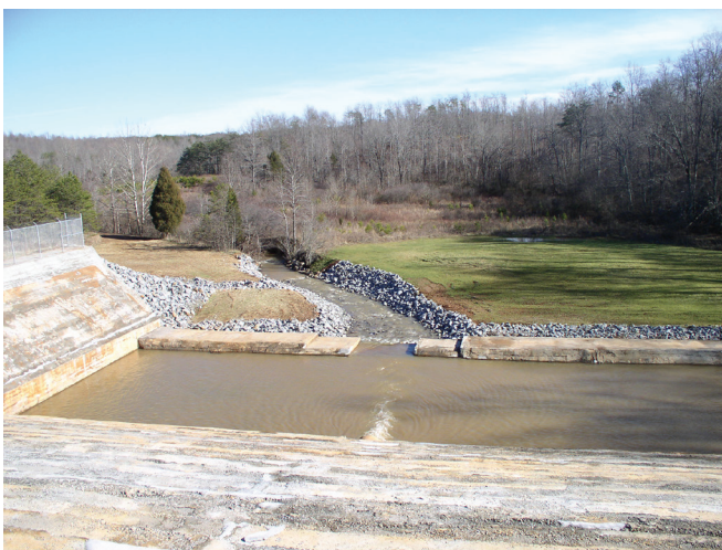
FIGURE 10-8. Damaged RCC surface.
