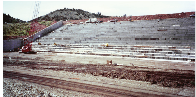
FIGURE 9-24. Precast CVC panels used for vertical step faces (Tongue River Dam, MT).
