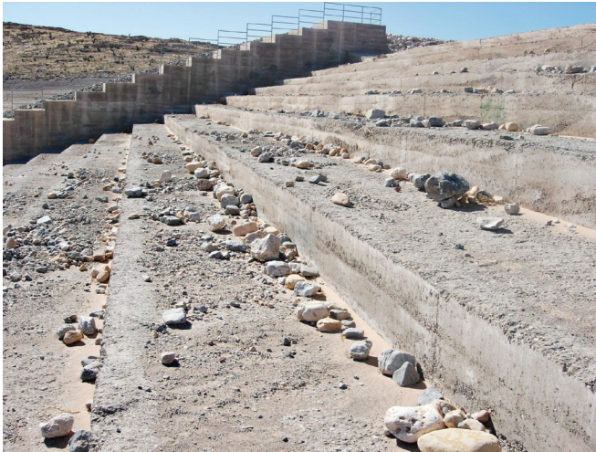
FIGURE 10-7. Debris on steps after flood event with very little loss of RCC material (Red Rock Basin, NV).
