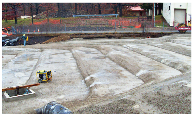
FIGURE 6-10. Unformed RCC chute with compacted RCC (Picati Lake Dam, NJ), courtesy of KC Construction.
