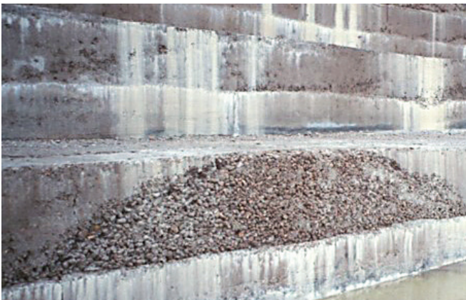
FIGURE 9-23. Poor RCC face.
