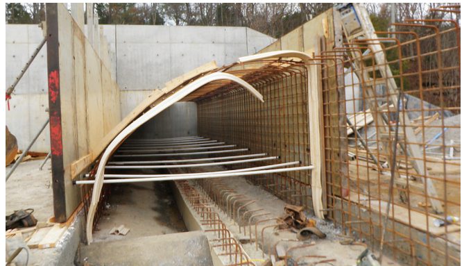
FIGURE 6-20. Side view of installation of reinforcement for ogee crest weir (Fox Creek MPS No.4, KY).
