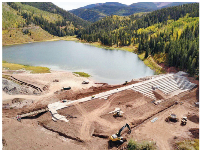
FIGURE 6-50. RCC spillway with topsoil cover placement in progress (Sylvan Lake Dam, CO).
