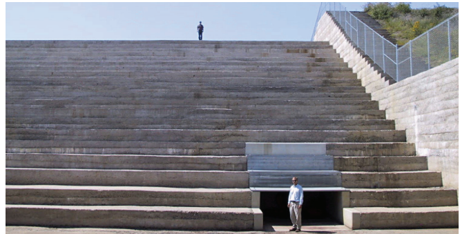
FIGURE 6-43. Vertically formed RCC training walls (East Fork Above Lavon 3C, TX), courtesy of Dennis Clute.
