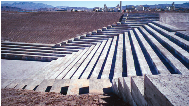
FIGURE 6-42. Formed sloped RCC training walls with deflection blocks to prevent erosion (Anthem Dam, NV).
