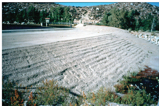
FIGURE 10-1. Loose aggregate after 10 years in service (Bishop Creek Dam, CA).
