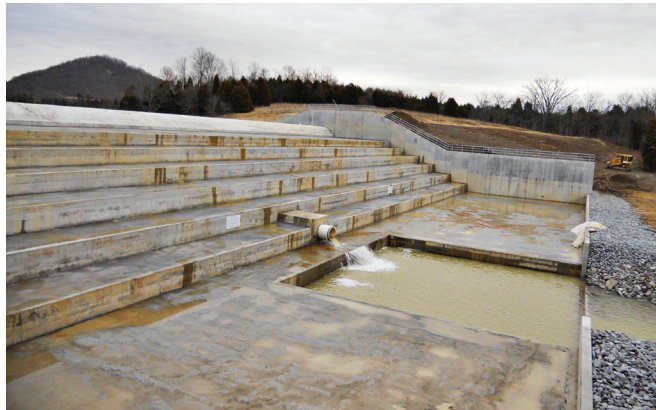
FIGURE 6-27. Run-out apron, end sill and riprap transition (Fox Creek MPS No. 4, KY).
