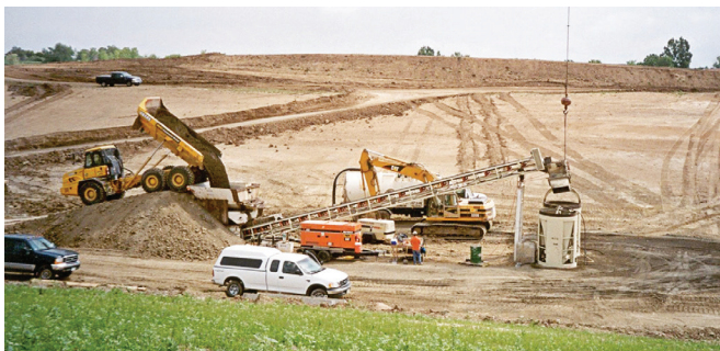
FIGURE 9-10. RCC loaded into concrete bucket to be delivered to placement area via crane.
