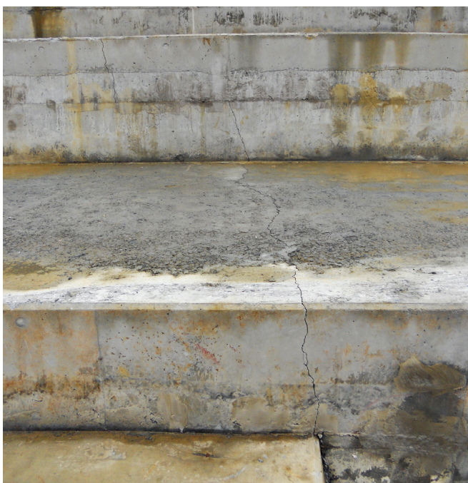
FIGURE 6-34. Naturally occurring shrinkage crack in RCC.
