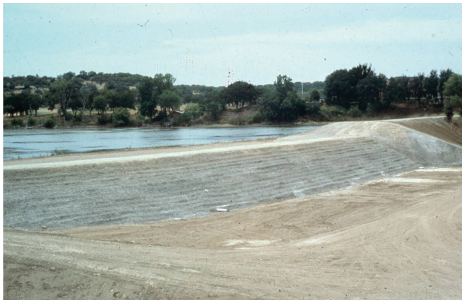
FIGURE 9-19. Unformed, uncompacted RCC steps.
