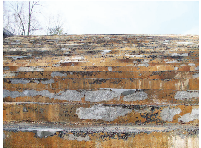
FIGURE 10-9. Damaged and poorly-patched RCC surface.
