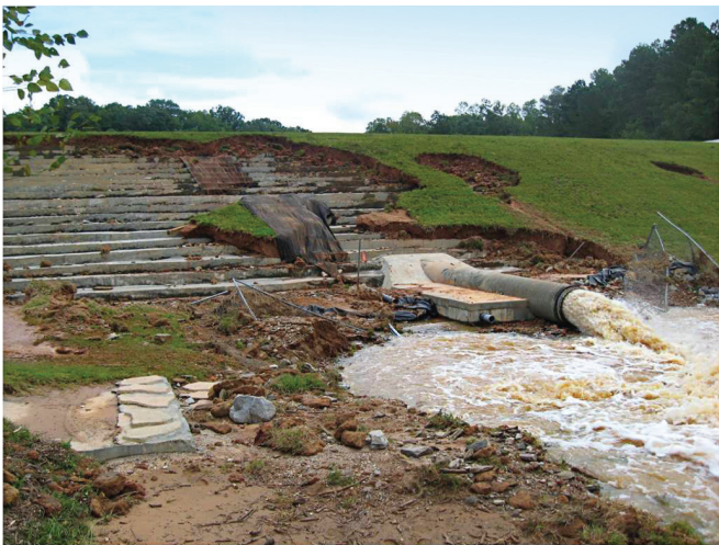
FIGURE 10-4. Overtopping spillway immediately after 2009 flood (Yellow River Structure Y-16, GA).
