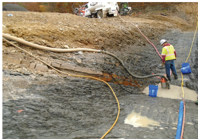
FIGURE 9-1. Dewatering sump adjacent to downstream cut-off wall in stilling basin runout apron.
