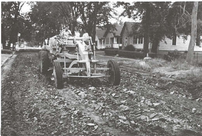
Ripping up old asphalt in preparation for recycling into soil-cement, Peoria, Illinois
