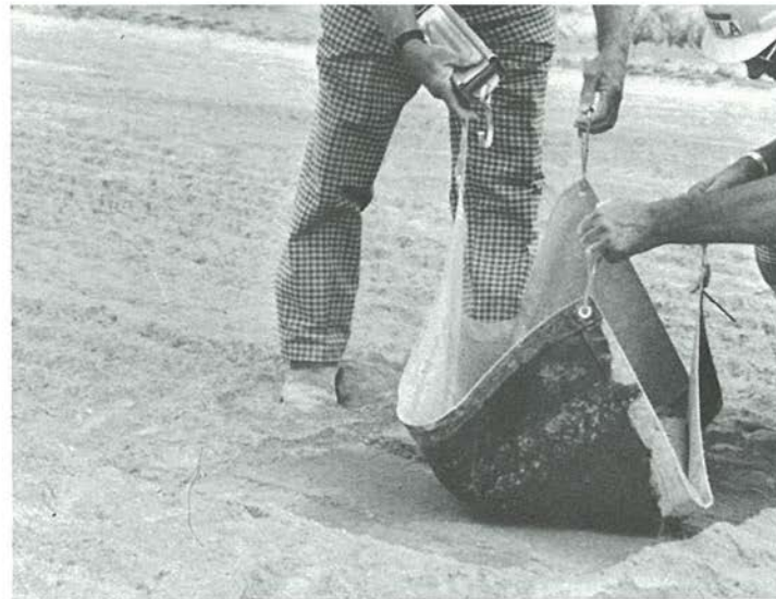
Fig. 8. Weighing cement collected on a square yard ( \text{m}^2 ) of canvas is a check on the quantity of cement spread.
