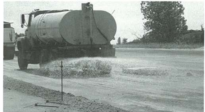
Fig. 28. Water truck applies light water spray to soil-cement surface to maintain moisture throughout compaction, finishing, and curing operations.
