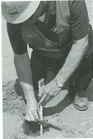
Fig. 27. Measuring depth of treatment through the density hole. A phenolphthalein solution can be squirted down the side of a freshly cut face of newly compacted soil-cement. The soil-cement will turn pinkish-red while the untreated subgrade material will retain its natural color.
