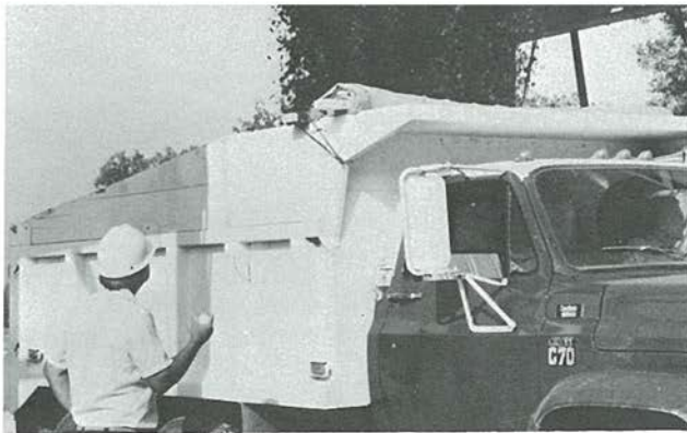
Fig. 10. Soil material is collected in a truck to determine rate of feed.
