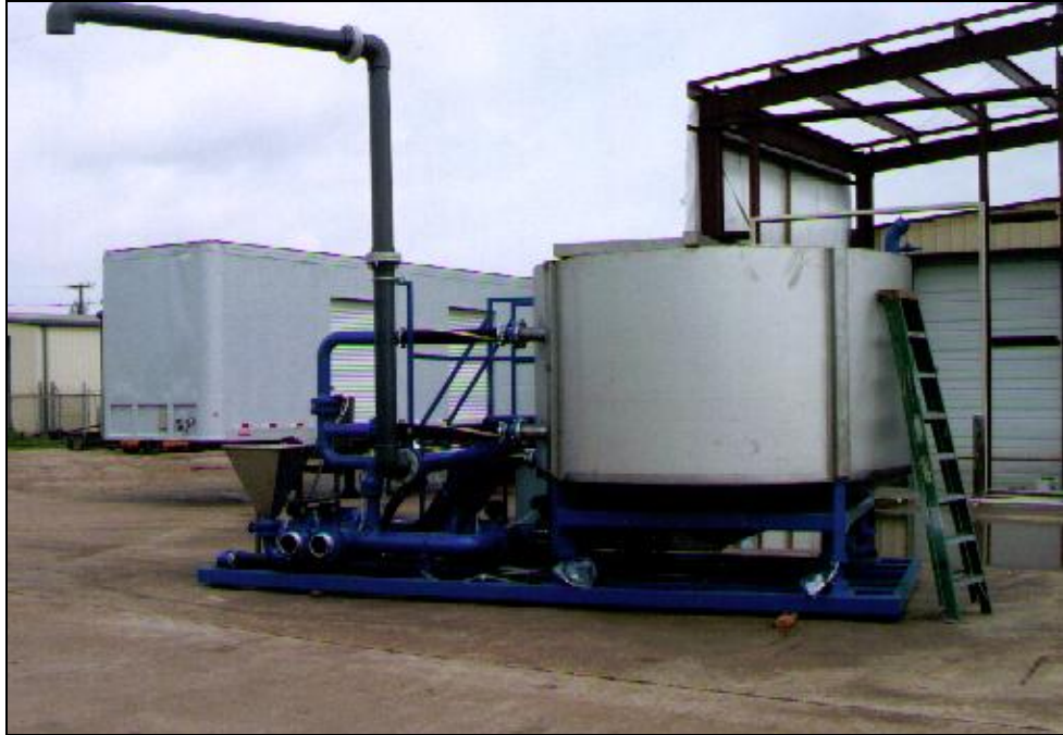
Figure 1.9. Texas Slurry Batch Plant.
