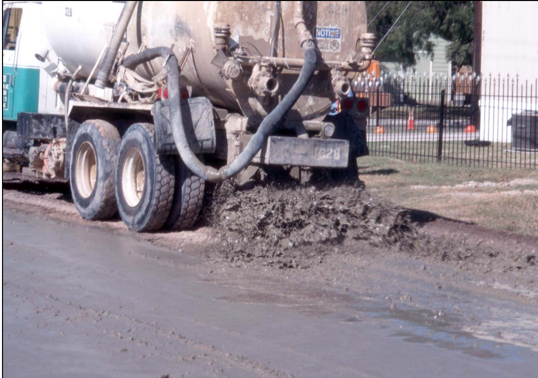
Figure 1.5. Spreading Slurry with the Olmos Construction Slurry Truck. Note: Photo courtesy of Olmos Construction.
