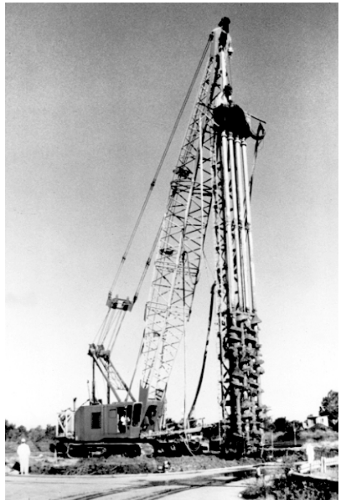
Fig. 1. Stabilization of wastes in situ using a specially developed soil mixing technique. (Courtesy of Geo-Con, Inc.)
