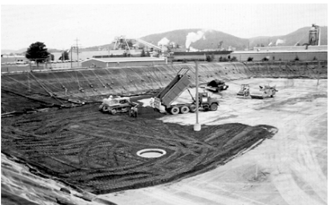
Fig. 3. Soil-cement used to line bottom of industrial wastewater storage lagoon. (Courtesy Solid Seal Systems)
