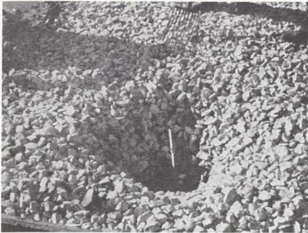
Fig. 39. A hole in the ballast gives assurance that grout is penetrating voids in the stone completely. Reference 5.
