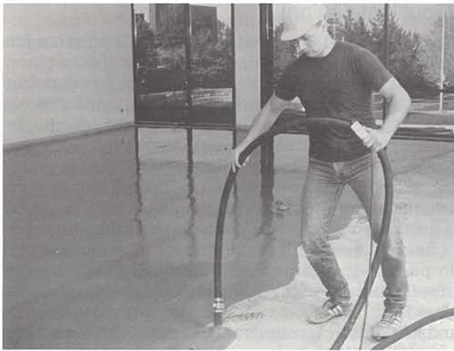
Fig. 21. Self-leveling floor toppings and underlayments are very fluid grouts that are easily placed by small-line pumps.
