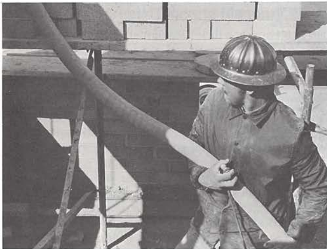
Fig. 16. While helping to handle the grout hose, a laborer controls the pump shutoff with a hand button. Reference 73.
