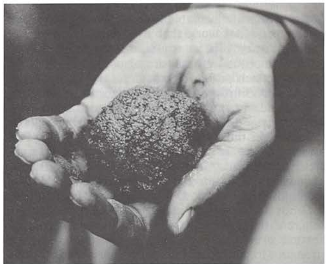
Fig. 23. A mixture of cement, sand, and just enough water to form a ball when compressed in the hand makes a good low-shrink mixture to repair or fill voids in concrete. This mixture is referred to as dry-pack mortar or dry-pack grout.
