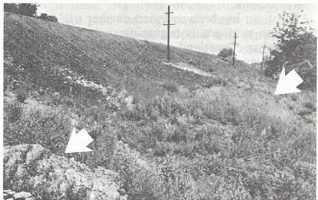
Fig. 42. The bulges on the fill slope of this railway roadbed show presence of water pockets. Reference 12.
