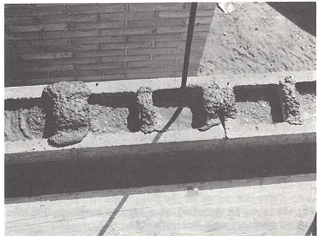
Fig. 18. Grouting is stopped about 1 in. below the top of the block to form a key with the next lift. Reference 73.
