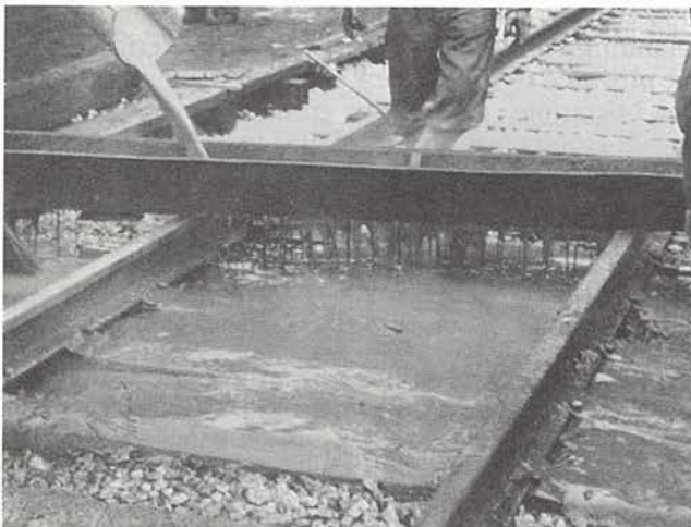
Fig. 40. Grout is deposited into the stone ballast by use of a trough that is moved forward as voids in the ballast become filled with grout. Reference 5.
