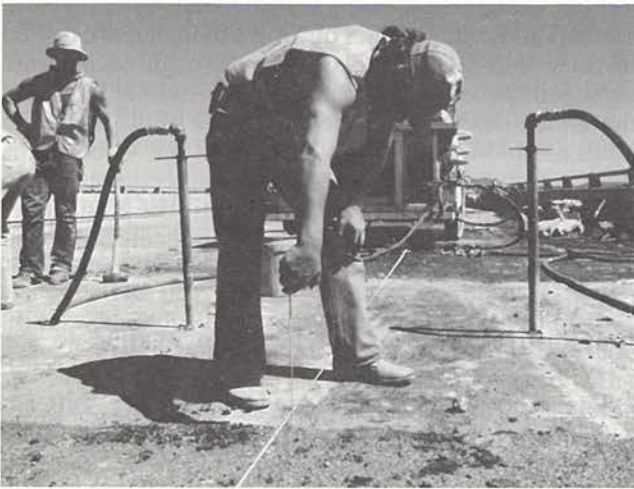
Fig. 31. Bridge approach is raised 5\frac{1}{2} in. in typical slabjacking project. Observe stringline and block used to control final elevation of slab.
