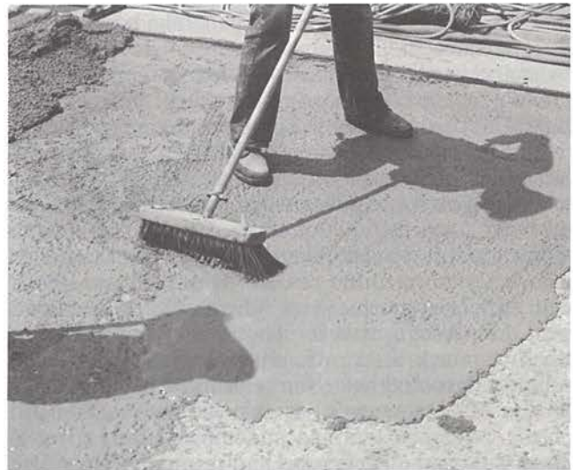
Fig. 22. Application of a bonding grout a few feet ahead of overlay concrete. The grout must not dry before the concrete is placed.
