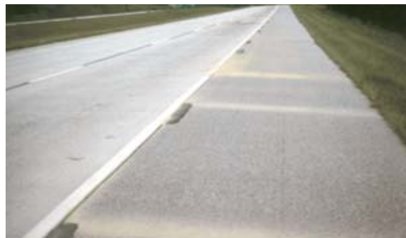
Figure 29. Stains on shoulders due to pumping.
