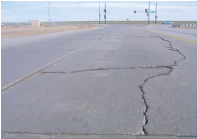
Figure 34. Example of a concrete pavement failure due to inadequate compaction of the subbase.
