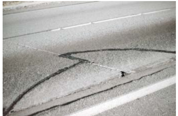
Figure 31. Corner break from void under corner of concrete slab.
