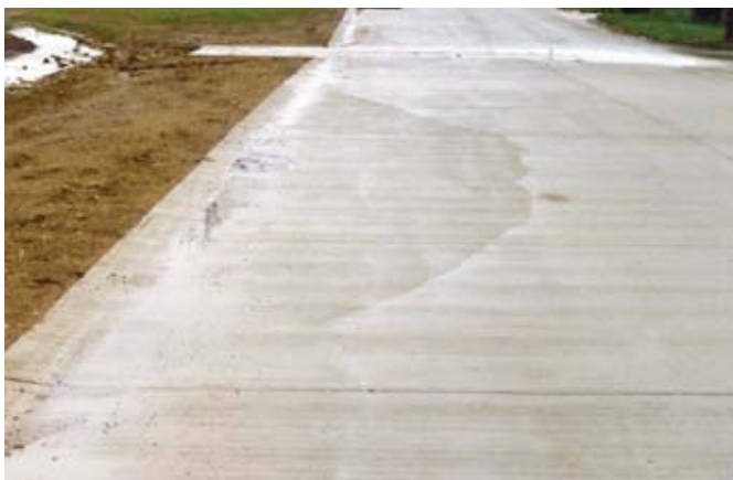
Figure 20. Common edge-to-edge crack attributable to differential frost heaving.
