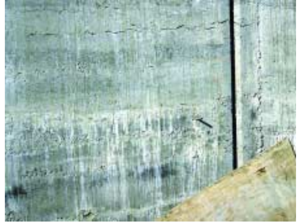
Figure 2.4. Formed RCC (above average quality) Bullard Creek Dam, OR, (photo courtesy of Benjamin Doerge).
