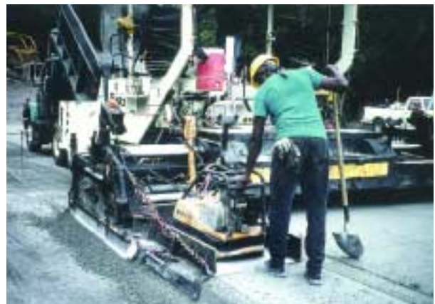
Figure 3.12. Paving machine and attachment used to form 9-inch-high steps at Woody Branch Dam, TX.
