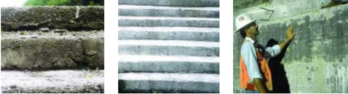
Figure 3.8. Examples of formed RCC steps of poor, fair, and good quality (left to right).
