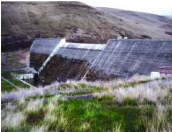
Figure 3.4. Seepage from downstream face, Willow Creek Dam, OR.
