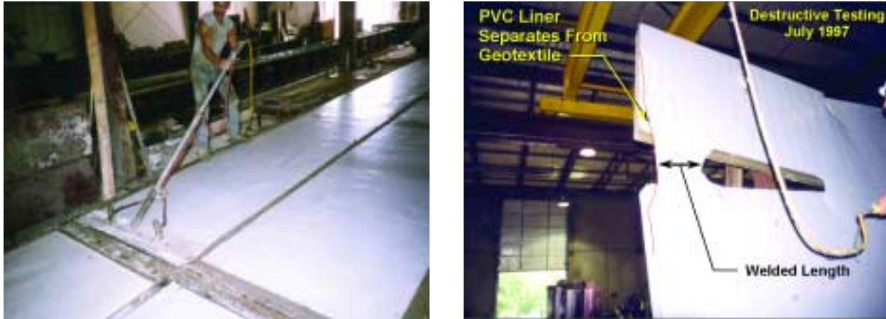
Figure 2.19. Photographs showing casting of precast panels with internal liner (left) and destructive testing of liner weld between two precast panels for Penn Forest Dam, PA.
