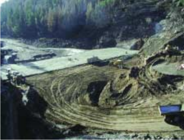
Figure 2.35. Earth fill placed concurrently with RCC at upstream face of Pajarito Dam, NM (photo courtesy of Terrence Arnold).
