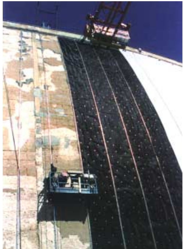
Figure 2.1. Installation of drainage layer to create fully drained face, (photo courtesy of CARPI).
