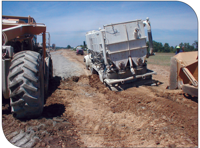
Figure 1 – Weak materials evidenced during modification
