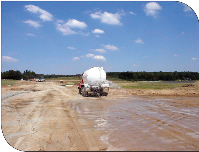
Figure 3 – Stability is apparent with little rutting under the weight of a water truck
