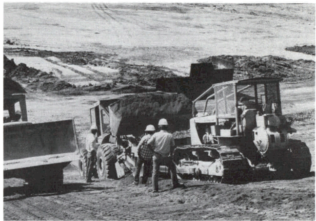
Fig. 13. Spreader running down the 3:1 slope places 12-in.-thick (300-mm) layer of soil-cement for spillway inlet channel at Palmetto Bend Dam, near Edna, Texas. Bulldozer at left is compacting soil-cement.
