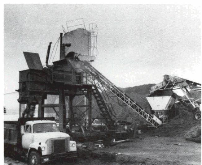
Fig. 1. Continuous flow central mixing plant. Note vibrating screen for removing oversized material.
