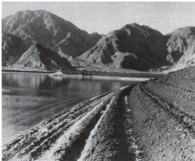
Fig. 6. Lake Cahuilla, Coachella County Water District, Calif. Two-ft-thick (0.6-m) soil-cement, constructed in stairstep fashion, protects embankment.
