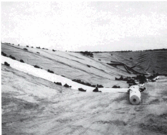
Fig. 10. Placing geomembrane over geotextile and 12-in.-thick (300-mm) soil-cement slope at Midland Terminal Reservoir, Texas.
