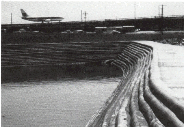
Fig. 8. Soil-cement lined pond for storing ethylene glycol runoff at Stapleton Field, Denver, Co.
