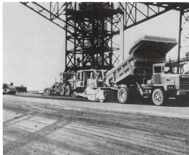
Fig. 11. Aggregate spreader being used to place central plant mixed soil cement for coal storage area at Independence Power Plant, near Newark, Ark.
