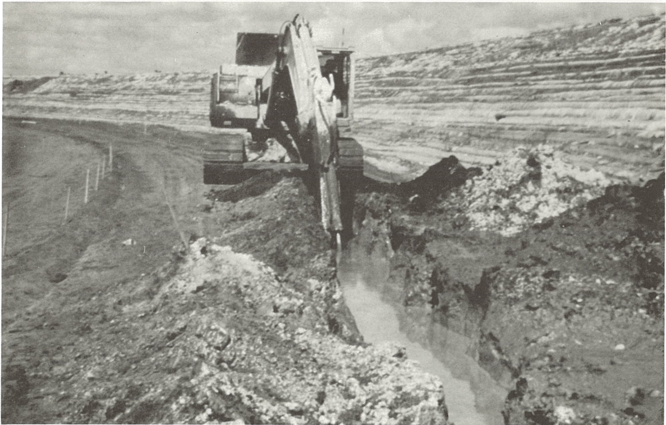
Fig. 1. Constructing cement-bentonite slurry trench along interior toe of slope for cooling water reservoir at Martin Power Plant, Fla. Note soil-cement slope protection in background.
