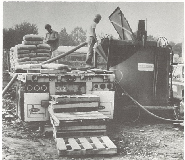
Fig. 6. Five-cu-yd capacity colloidal mixer. Vertical shaft with propellers located in center of tank assists slurry mixing. (Courtesy of Geo-Con Inc., Pittsburgh, Penn.)
