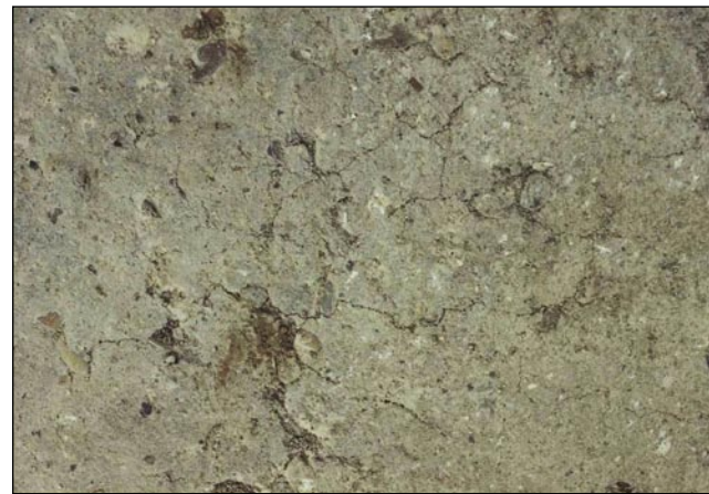
Visible cracks in CTB after microcracking are rarely observed.
