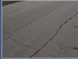
Block cracking typical of CTB.
