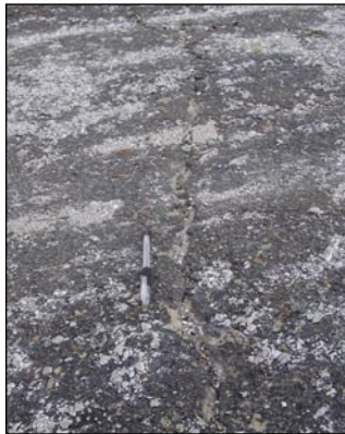
Crack in moist-cured section.
