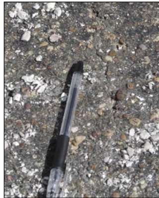
Crack in section microcracked.
