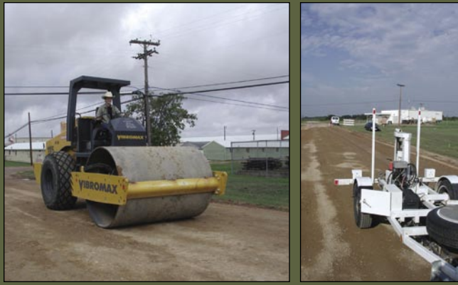
Microcracking in progress with the vibratory roller. TxDOT's FWD can serve as the control mechanism to determine when to stop rolling by measuring the reduction in average base modulus.
