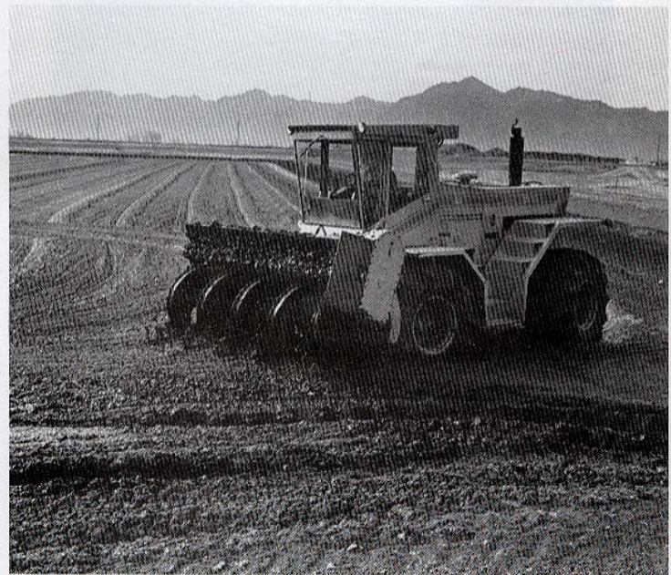
Mechanical mixer turns sludge over in newly constructed lagoon to accelerate drying.
