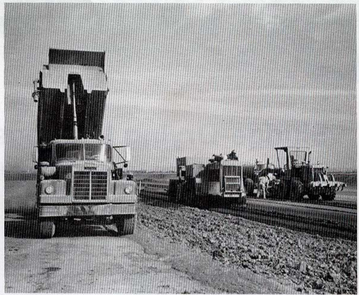
Soil-cement is constructed by mixed-in-place method along the bottom of the lagoon.
