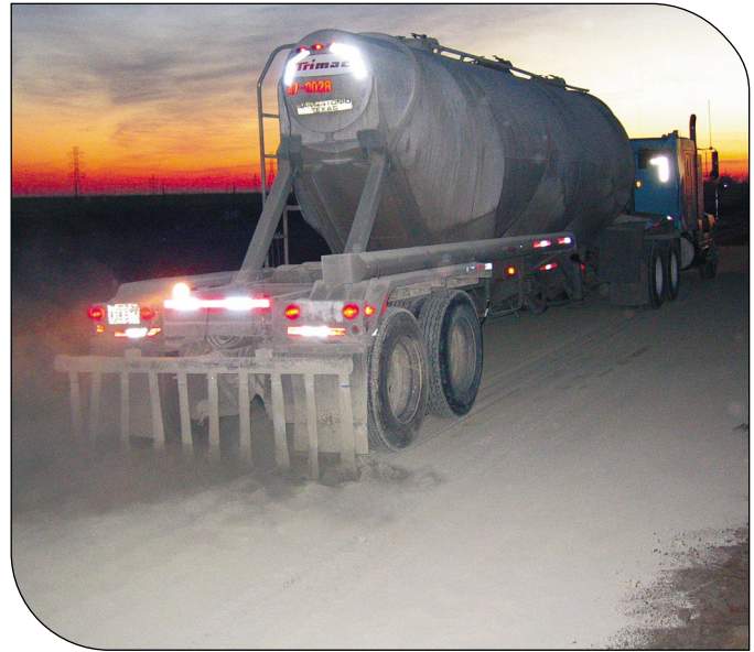
Cement is spread in a 37-ft by 388-ft lane marked off by Zachry crews.
