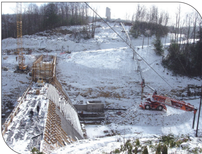
RCC mixing plant and conveying system. Photograph was taken during cold weather shutdown
