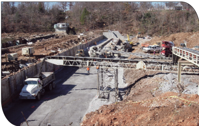
RCC conveying system
