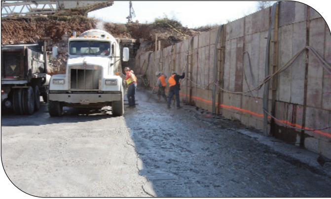
Spreading mortar to control seepage and bond RCC lifts downstream from facing concrete
