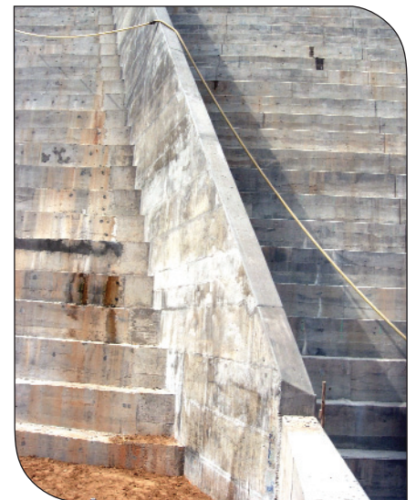
Training wall and steps showing conventional concrete on right and grout-enriched RCC on left.
