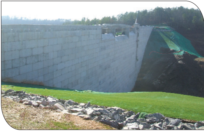
General view of upstream face of completed dam prior to initial filling.
