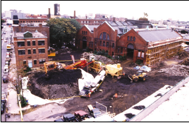
Figure 5. Ex situ S/S treatment of lead- and arsenic-contaminated soils in Boston, MA.
