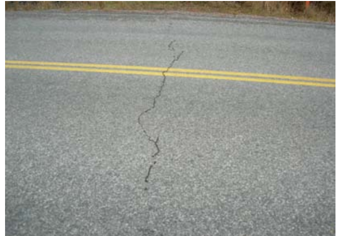
Figure 9. Reflection cracks on FDR with cement road, Stevens County, WA.
