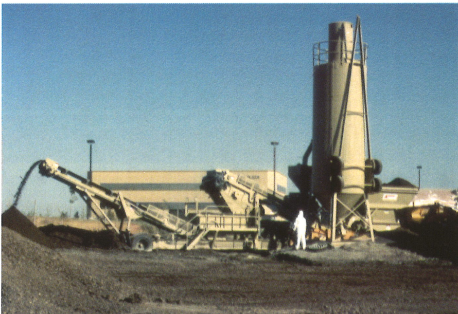
S/S treatment system from right to left—input hopper, portland cement/CKD (reagent) silo, belt conveyor with reagent feed controls, pugmill, belt conveyor, discharge of treated soil.
