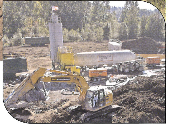
S/S binding reagent mixing plant.
