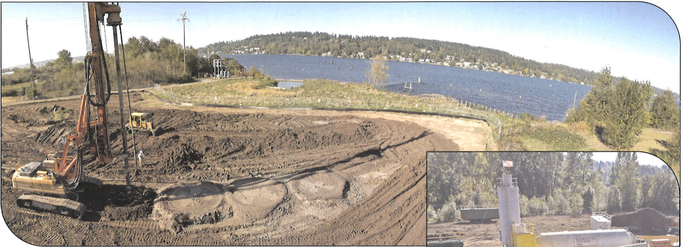
S/S at the Renton, WA, site.
